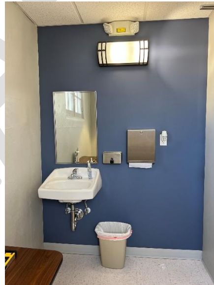
Unisex Restroom Sink
