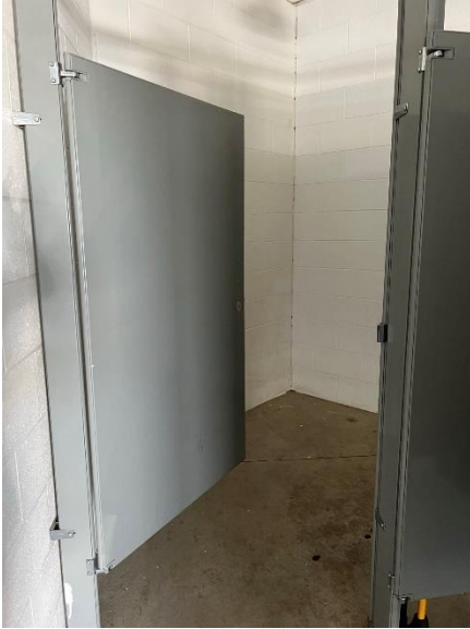
Women's Restroom Stall Door (1)
