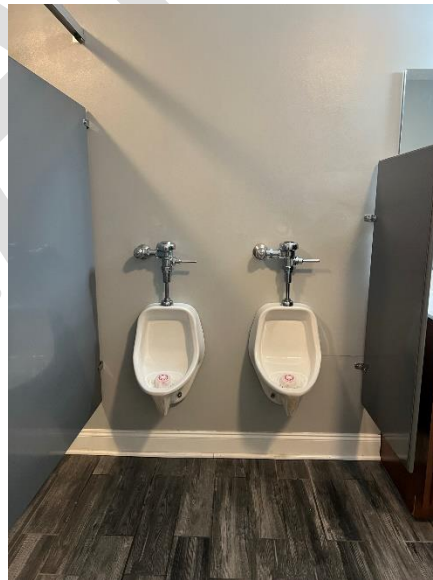
Men's Restroom Urinal
