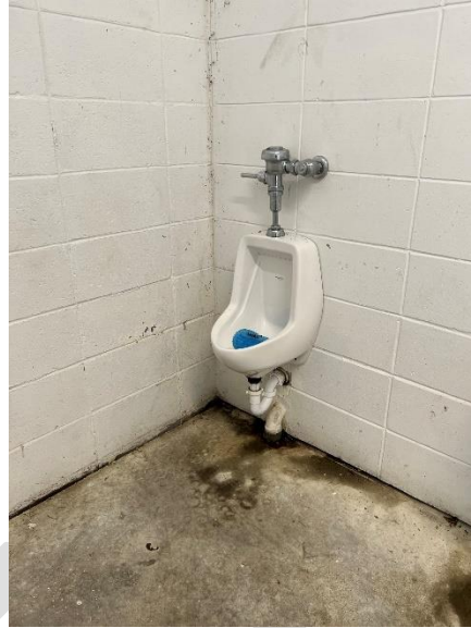
Men's Restroom Urinal (2)
