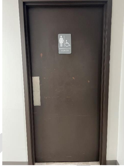
Women's Restroom Door (Ivy Tech)
