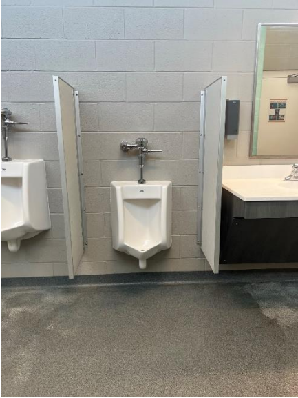
Men's Restroom Urinal
