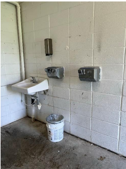
Men's Restroom Sink (2)
