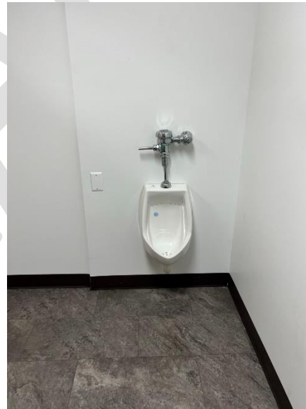
Men's Restroom Urinal (Ivy Tech)
