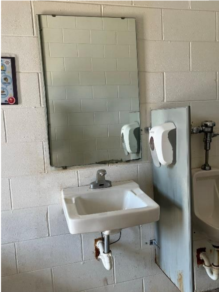
Men's Restroom Sink (1)
