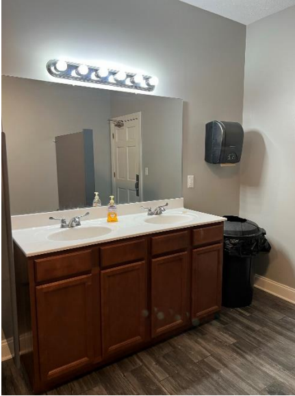
Men's Restroom Sink
