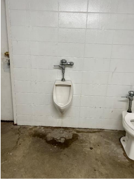
Men's Restroom Urinal (3)
