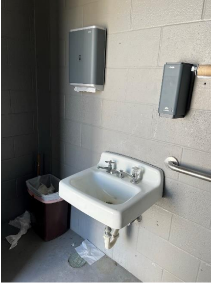
Unisex Restroom Sink
