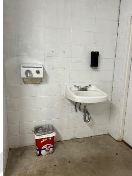
Men's Restroom Sink (3)
